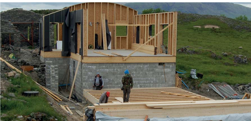
Main floor and western gable erected using 300A+ JJI-Joists, lower floor using 400C JJIs
