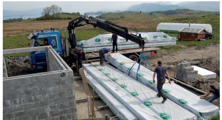
Unloading the 12m long JJI packages onto the foundations of the lower floor
